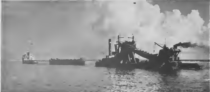
STEAMING OUT from the east end of the harbor is a little flotilla bound for Curacao. Towing the barge and excavating equipment used in dredging the harbor is an ocean-going tug from Rotterdam.
